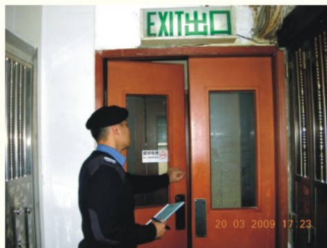
● 消防人員巡查舊式樓宇的消防安全 Fire personnel inspecting fire safety of old buildings
